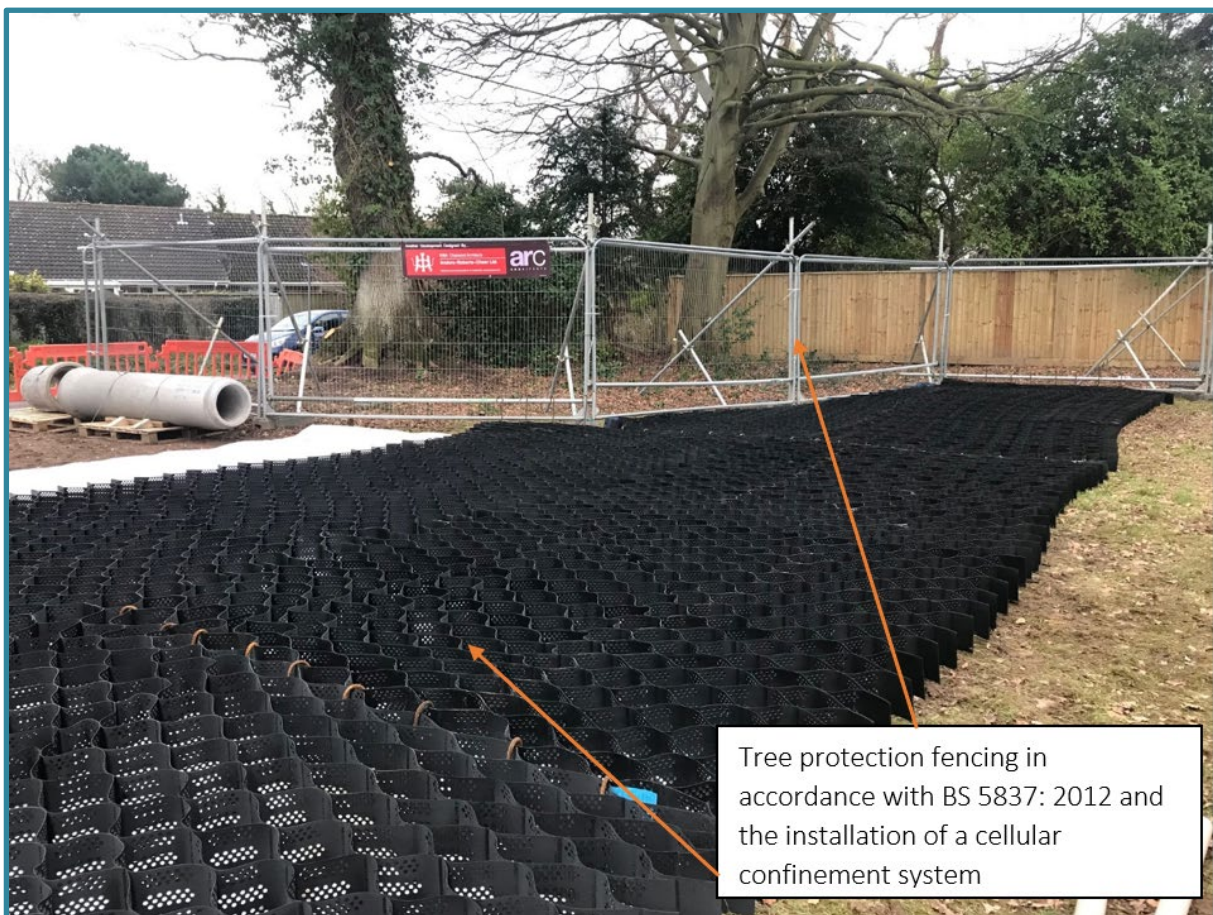
Figure 18. A 3D cellular confinement system, laid and secured with road pins and awaiting infill with washed angular stone to complete the ground protection and later to base the new driveway upon
