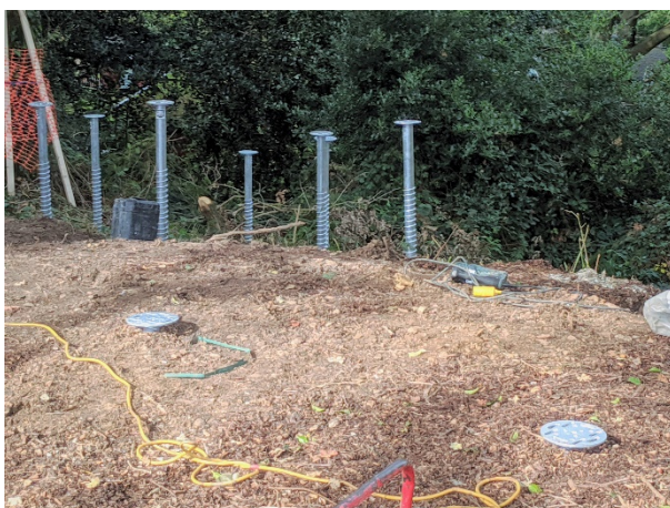
Figure 31. Less invasive screw piles being installed inside the RPA's of protected trees to support new structures
