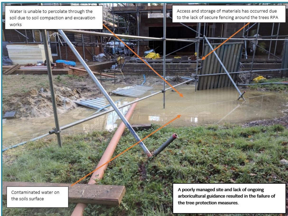
Figure 21. Failure to protect trees to be retained
